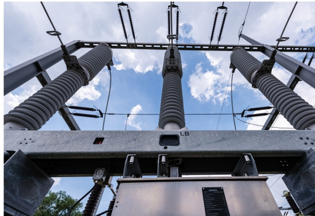
World's first substation with SF 6 -free switchgear technology from Siemens Energy in a 110 kV high-voltage grid (Noerdlingen, Germany 2018)
